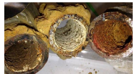
A view into Flint drinking water pipes, showing various types of iron corrosion and rust.
