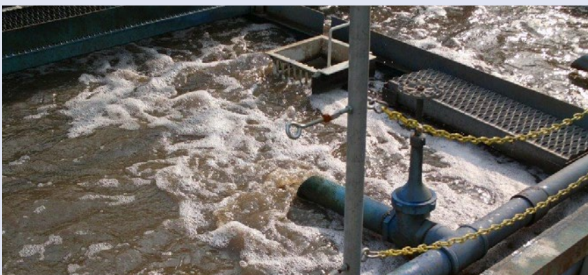
Example of activated sludge tank at a wastewater treatment plant.
