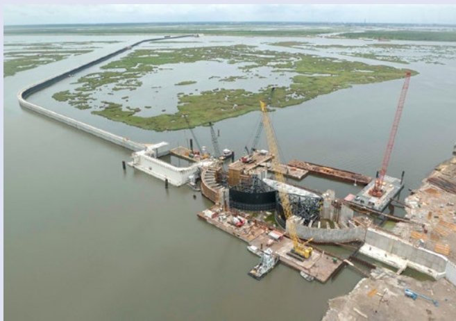
Construction of the massive New Orleans Inner Harbor Navigation Canal Surge Barrier (IHNC) at Lake Borgne, the largest design-build civil works project in USACE history.
