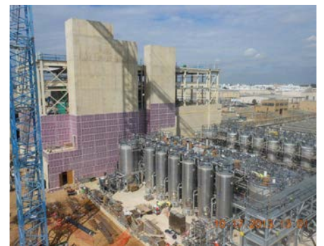
Cambi System (thermal hydrolysis) with the Pre-Dewatering Building in the background
