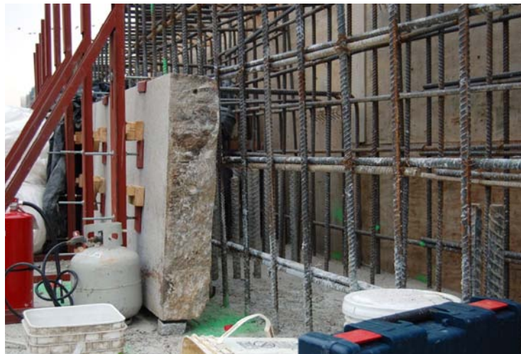
Original Ashlar facing stone re-positioned before pour of bottom section of the new wall stem.
