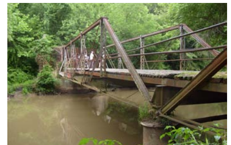
Queen Anne Bridge span, looking from Anne Arundel side toward Prince George’s County bank of the Patuxent River. Photo by BGD.
