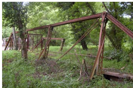
Queen Anne Bridge truss span on Anne Arundel County side. Collapsed under overload weight of a crossing truck. Photo by BGD.
