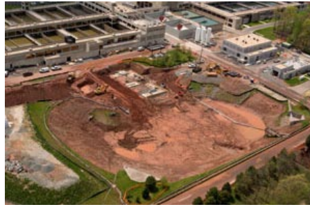
Aerial view of the Pond C improvements at the Corbalis Water Treatment Plant.
