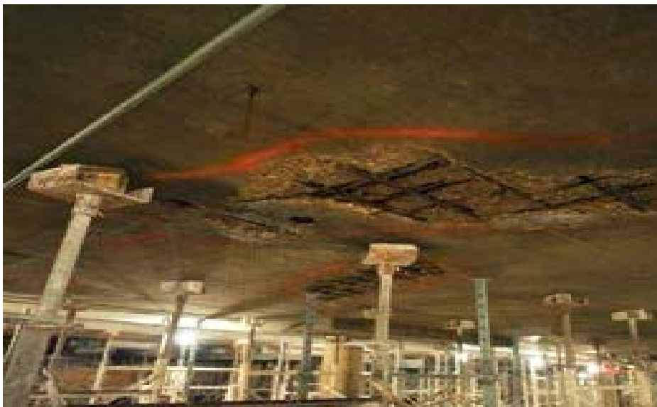
Deteriorated Soffit Areas Identified for Repair
